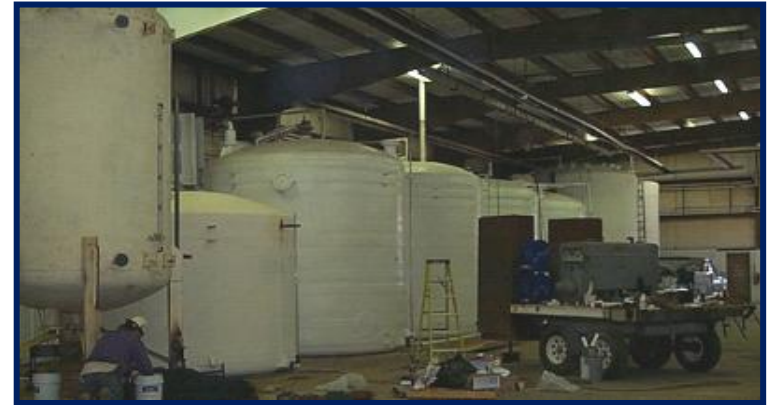
Irigaray Central Processing Facility
