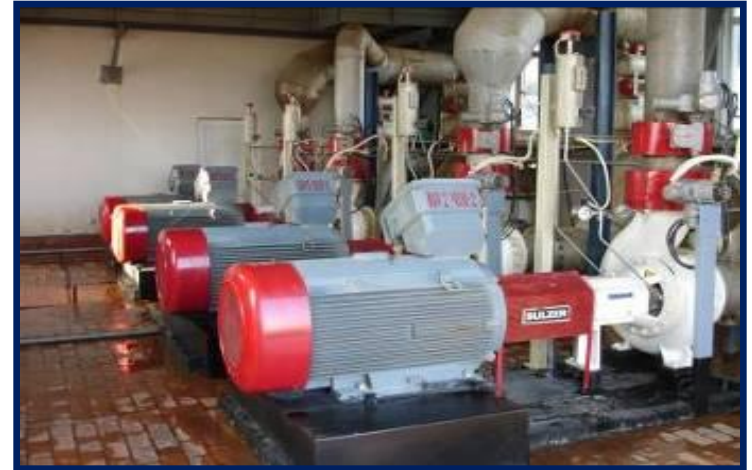
Pump House at Akdala
